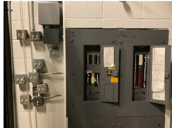
Stage Electrical Panels
